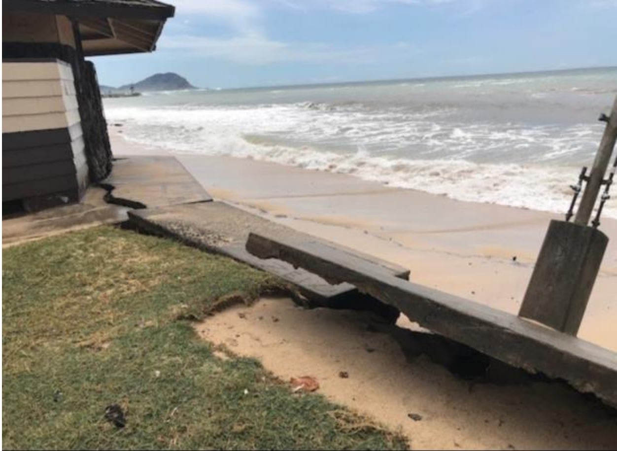
Figure 10: Destruction of Public Facilities, Maunalahilahi Beach Park, 2018
