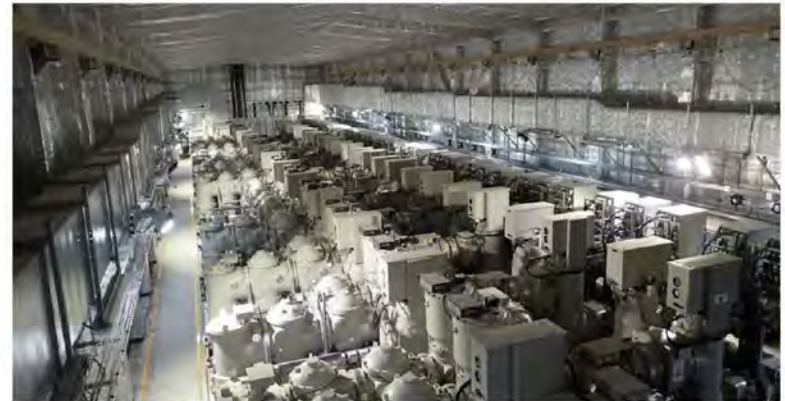
Inside of main substation
